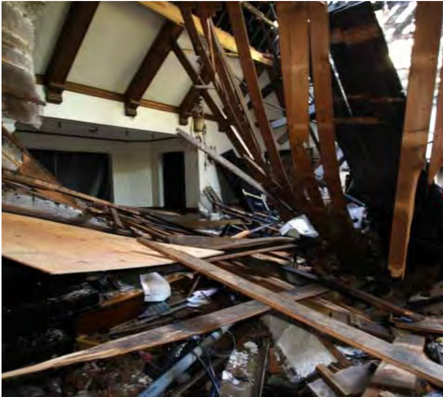
A look inside the auditorium after the fire at the Indian Boundary Park Fieldhouse on May 20, 2011, Photo Courtesy of Beth Martin
